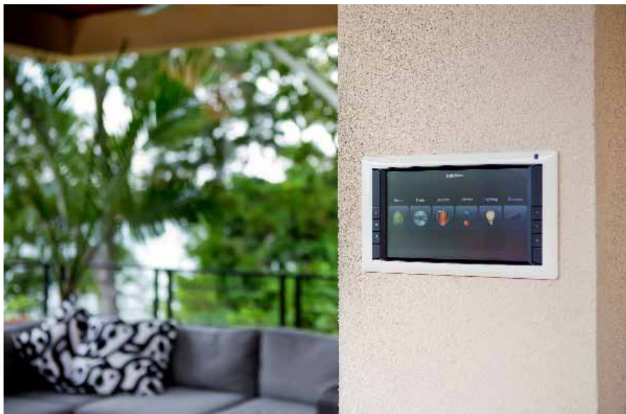
Outdoor control touchscreen installed by Sound Concept
